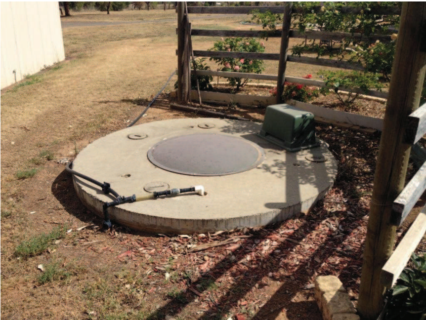
Plate 20: Septic System located within Lot 413 in DP 1003586
