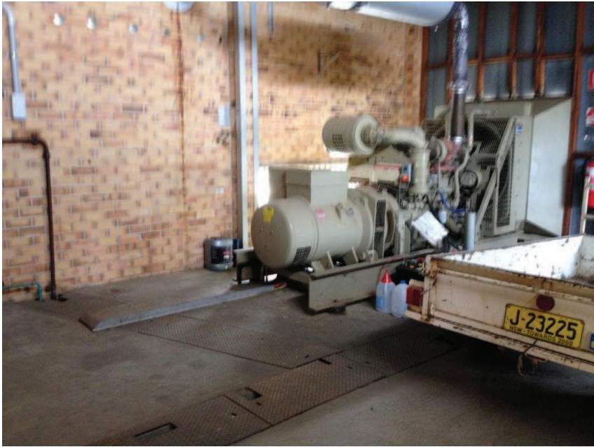
Plate 11: View of the Emergency Generator used by the Prime News Station
