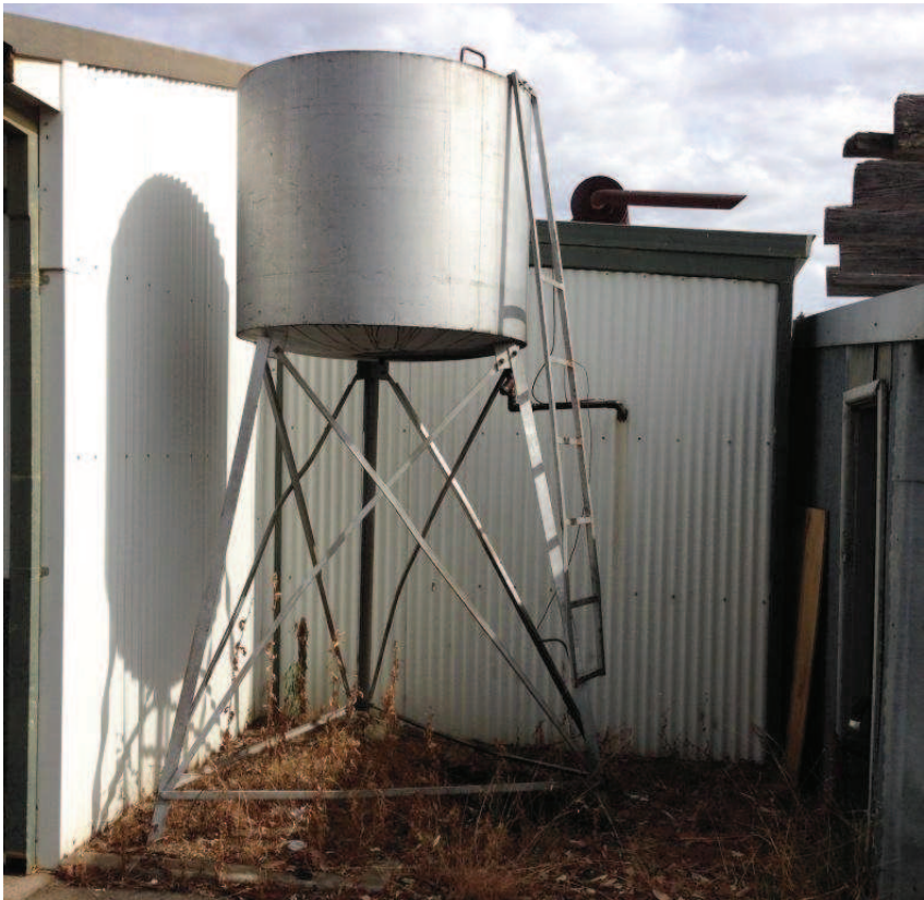
Plate 18: View of Above Ground Storage Tank in Lot 1 in DP 162623
